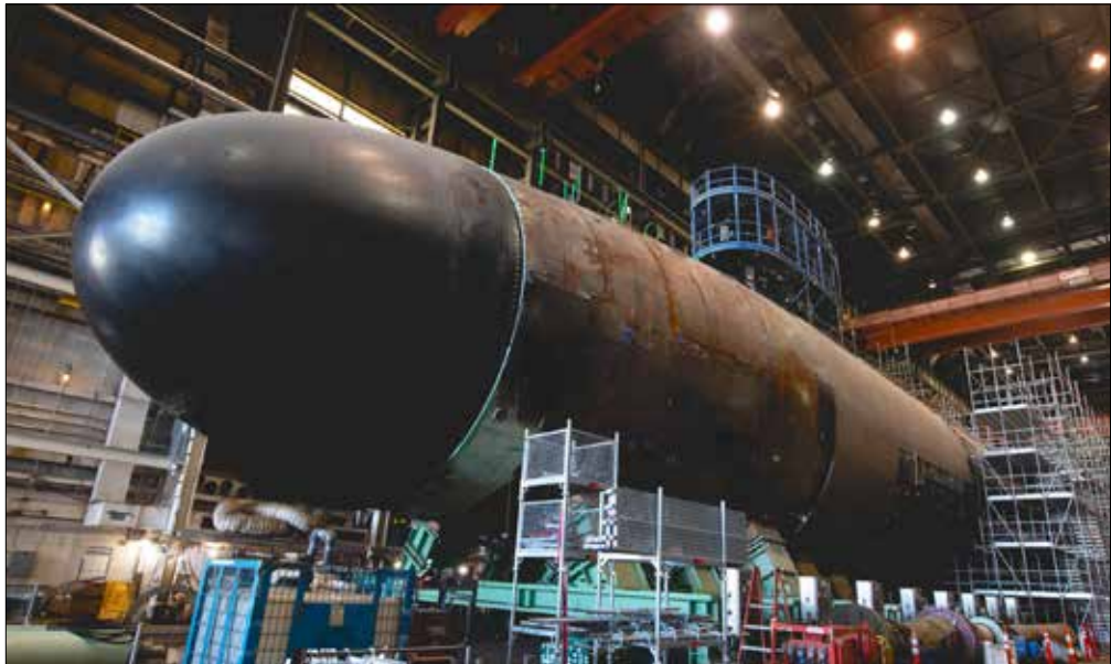
In-progress Virginia-class submarine USS Arkansas (SSN-800) as "pressure hull complete," meaning all her hull sections are now joined to form a single, watertight unit. (U.S. Navy photo.)
